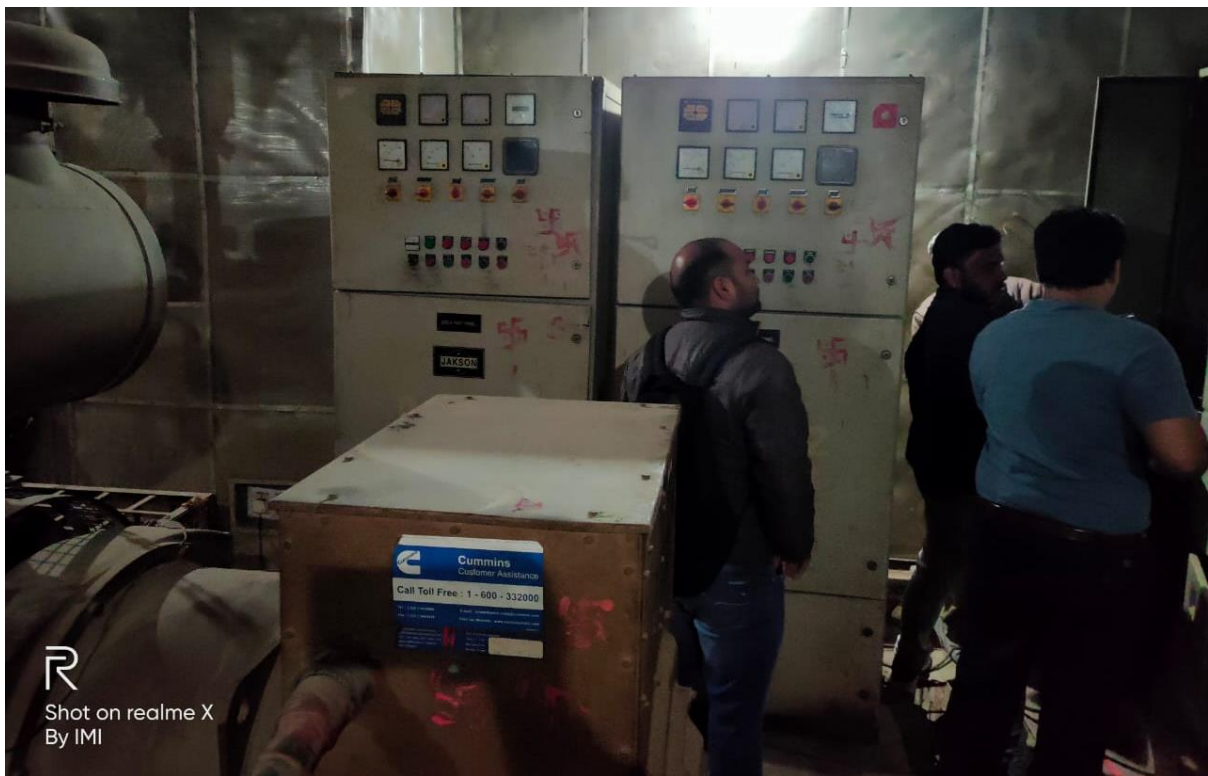
2 LT panels to which grid and DGs are connected
