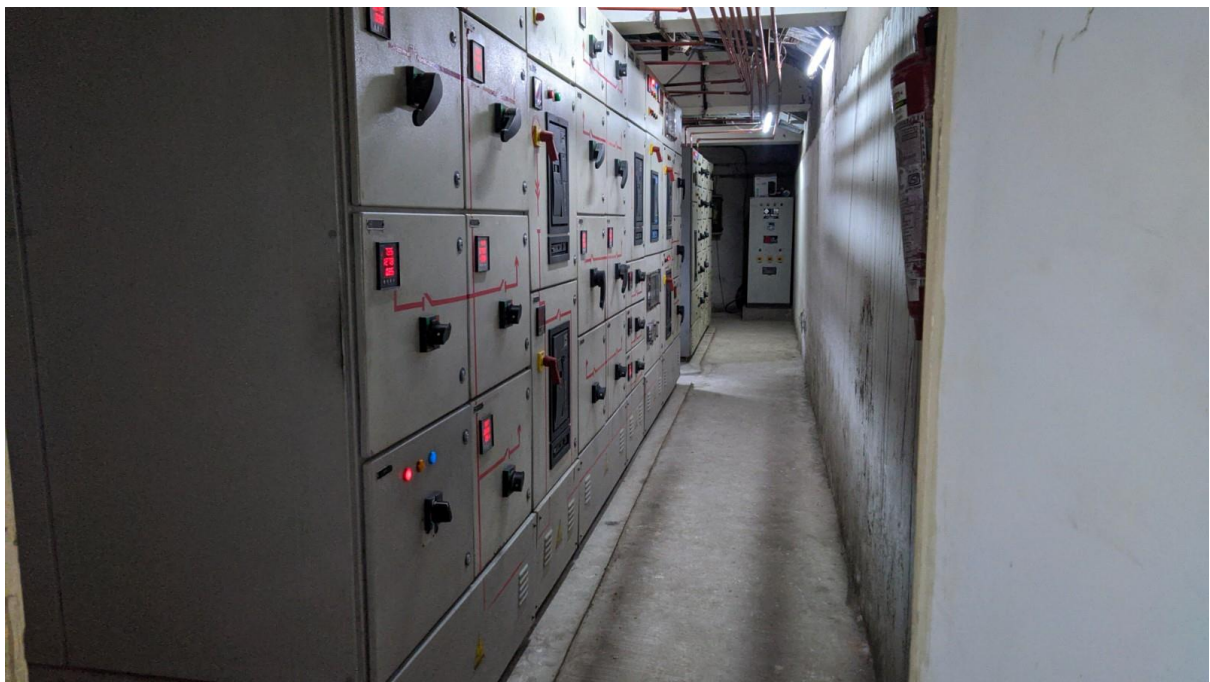
Inside view of LT Control Room
