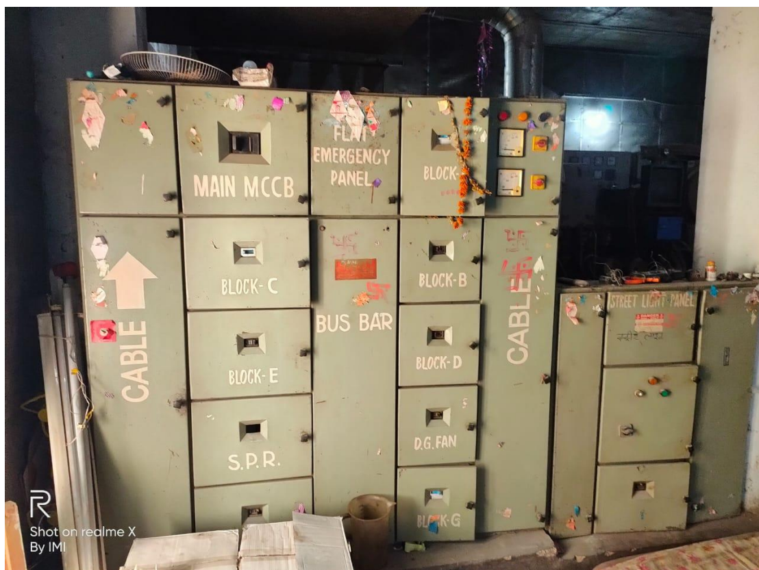
Set of LTDBs / ACDBs for lifts, pumps, house blocks
