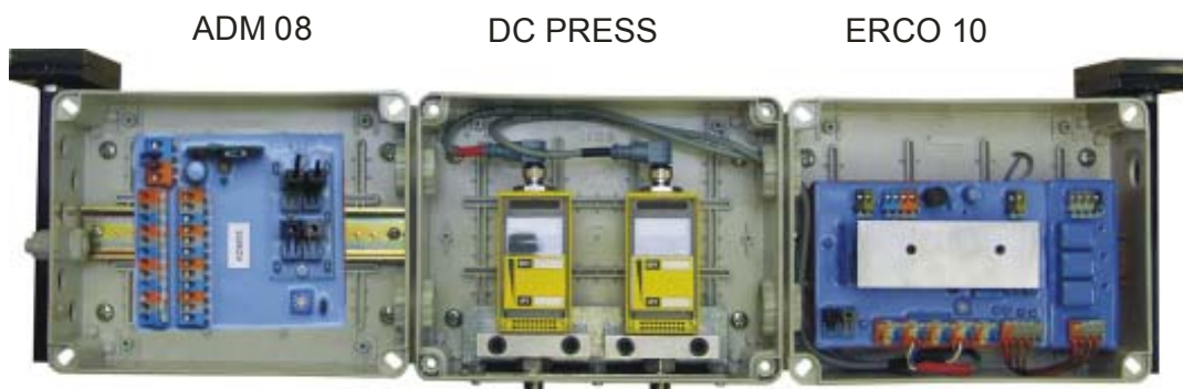
auxiliary switchboard left (PR1)
