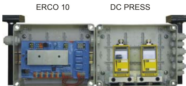
auxiliary switchboard right (PR2)
