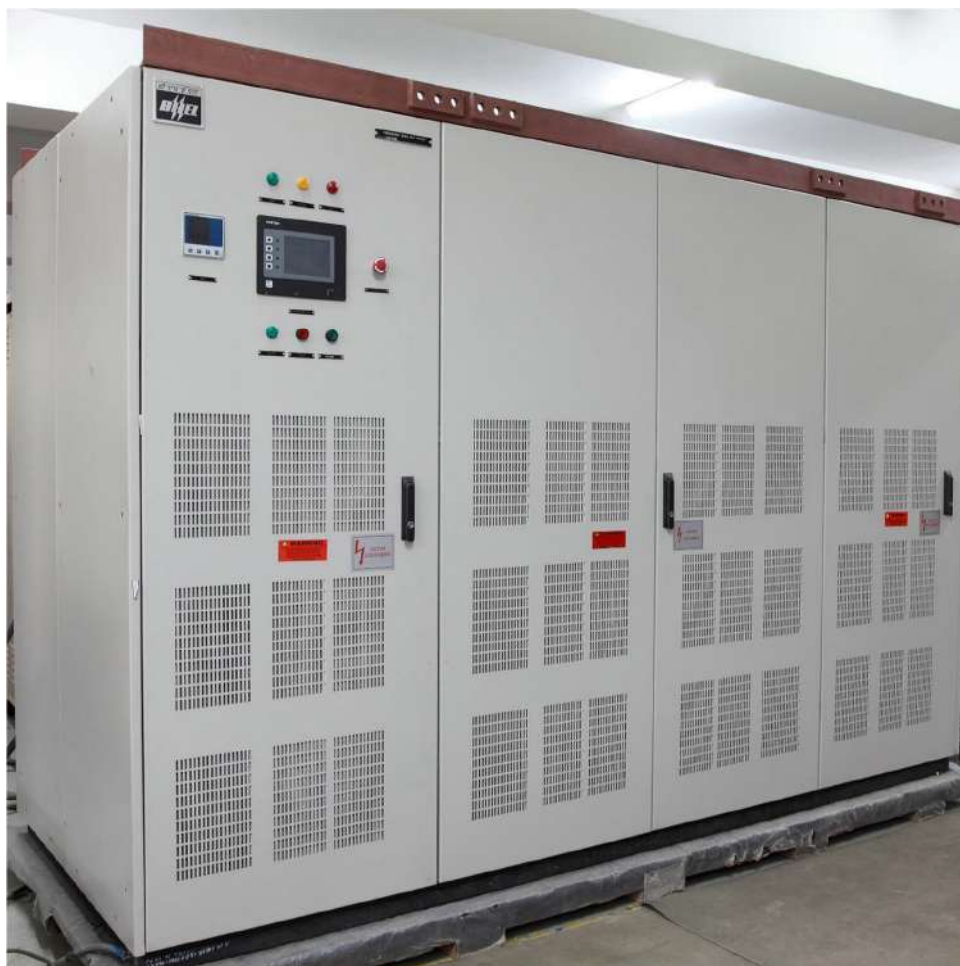
Front External View Of A 1.25MW PCU
