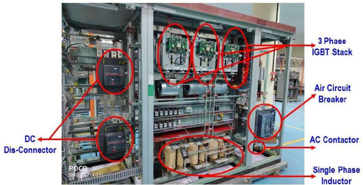
Front Internal View Of A 1.25MW PCU
