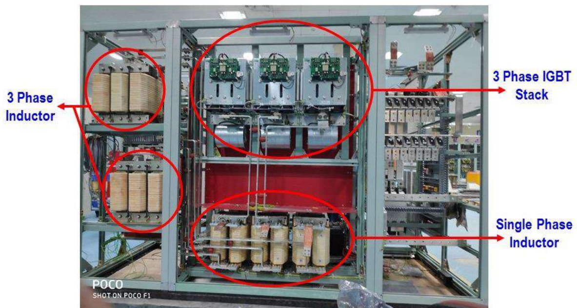
Rear Internal View Of A 1.25MW PCU
