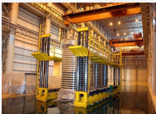
Transformers - Final Assembly Platform
