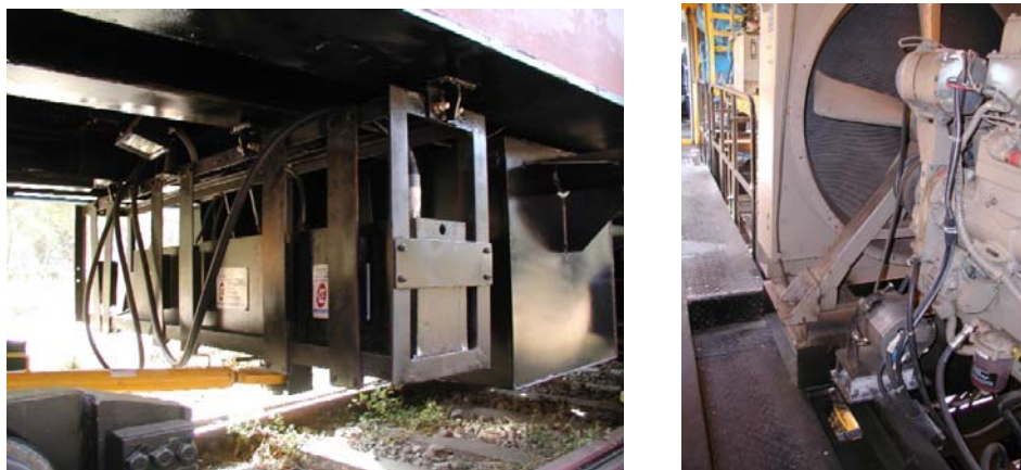
Fig. 11, 12 Battery arrangement and charging alternators
