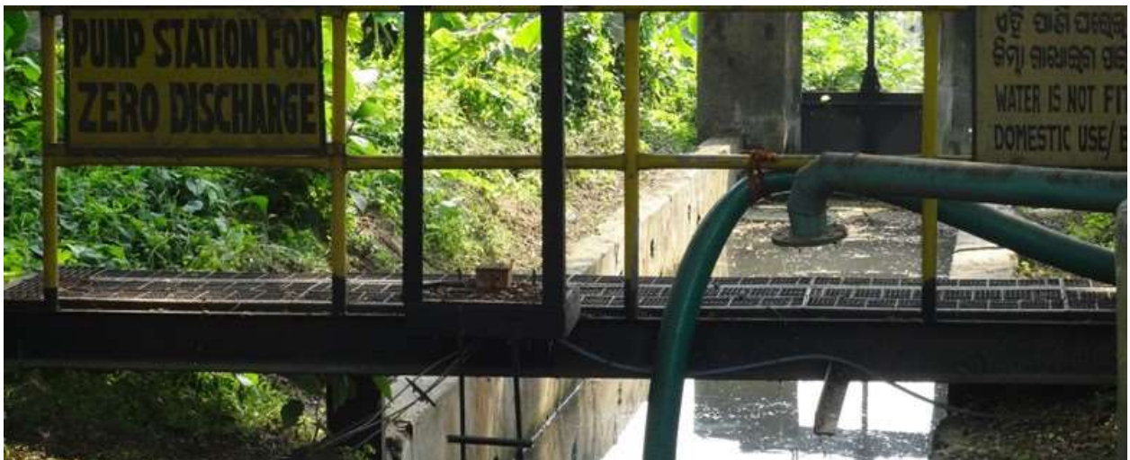
Photo 2.2: Effluent and storm water is pumped back for treatment as part of zero discharge plan
