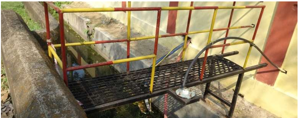
Photo 2.4: Drain Water pumping to STP as part of zero discharge plan
