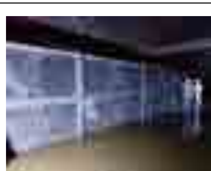
FRP grating in baffle wall
