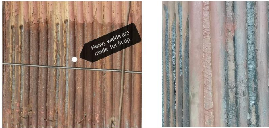
Figure-1 Photograph of excess welding on the fin
