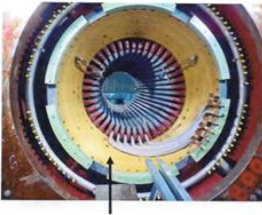
For support and consolidation of the overhang structure of large size TG (above 500 MW ratings).
