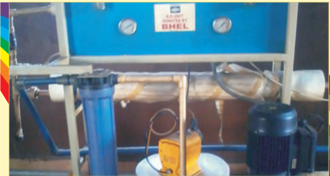
RO Plant for clean drinking water at Tuticorin Site
