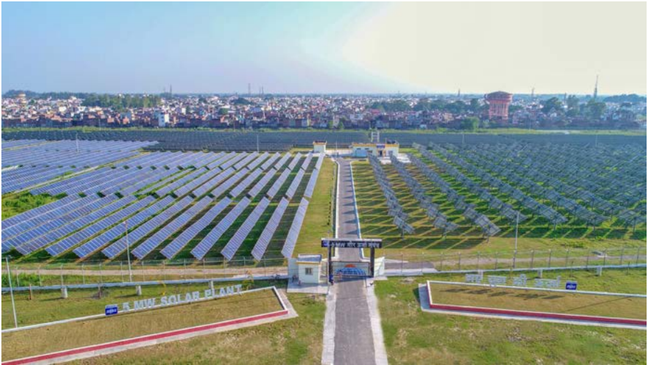
5 MW solar power plant including ground-mounted, fixed, motor tracking & passive tracking enabled modules of BHEL make at Haridwar plant premises
