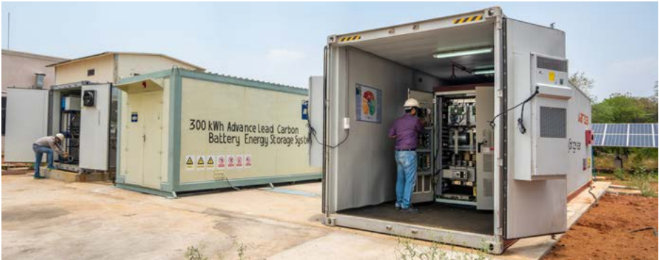
1 MW Battery Energy Storage System (BESS) for in-house usage, developed and commissioned at Corporate R&D, Hyderabad
