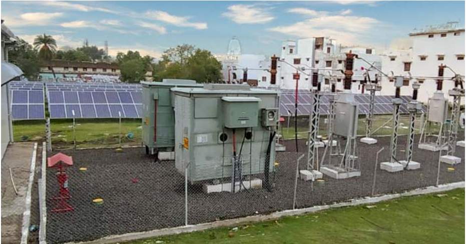
1.7 MWp Solar PV plant at Bina, Madhya Pradesh for Indian Railways commissioned by BHEL
