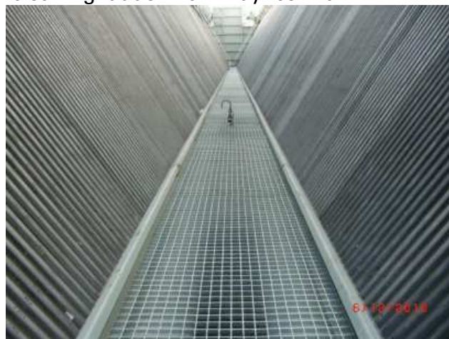
cleaning ladder walk way -central
