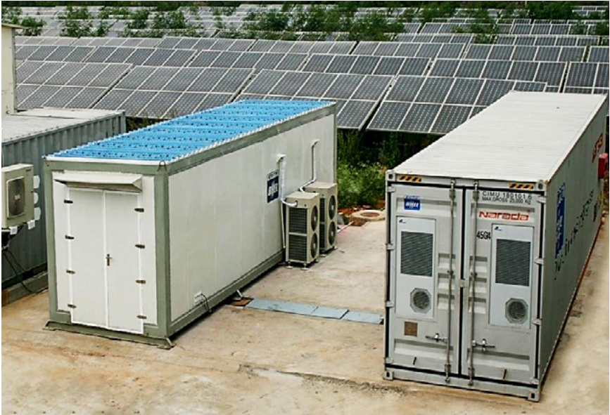
BHEL is executing its maiden order of setting up of a cumulative 410 kWh Battery Energy Storage Systems (BESS) for TERI
