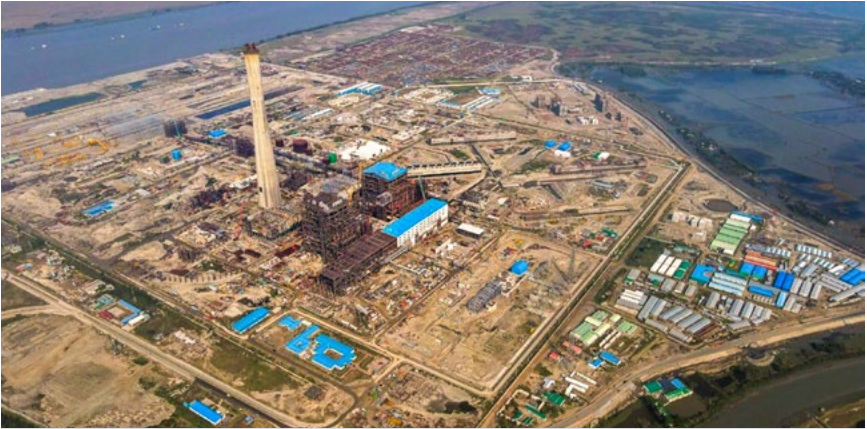
2x660 MW Maitree Supercritical Power Project being executed by BHEL in Bangladesh
