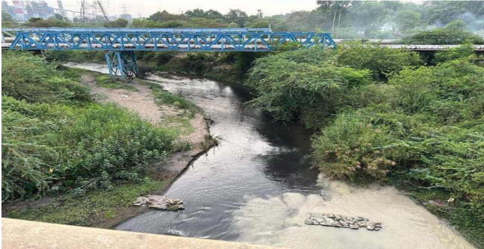
Figure 2.5 Ash slurry flowing into Balia nala due to leakage in the ash slurry pipe –view from road bridge on nala
